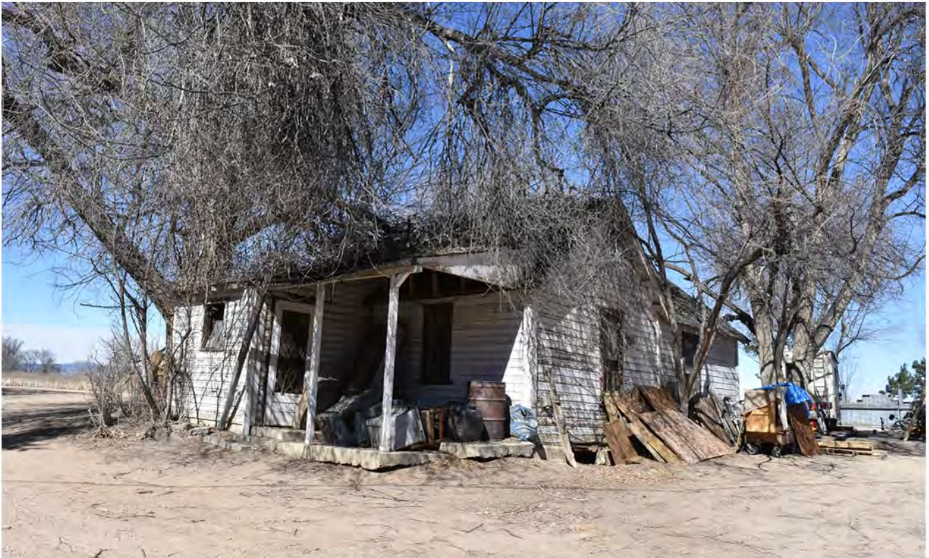
5LR14128_2: View northwest of the one-story secondary dwelling located west of the main house.
