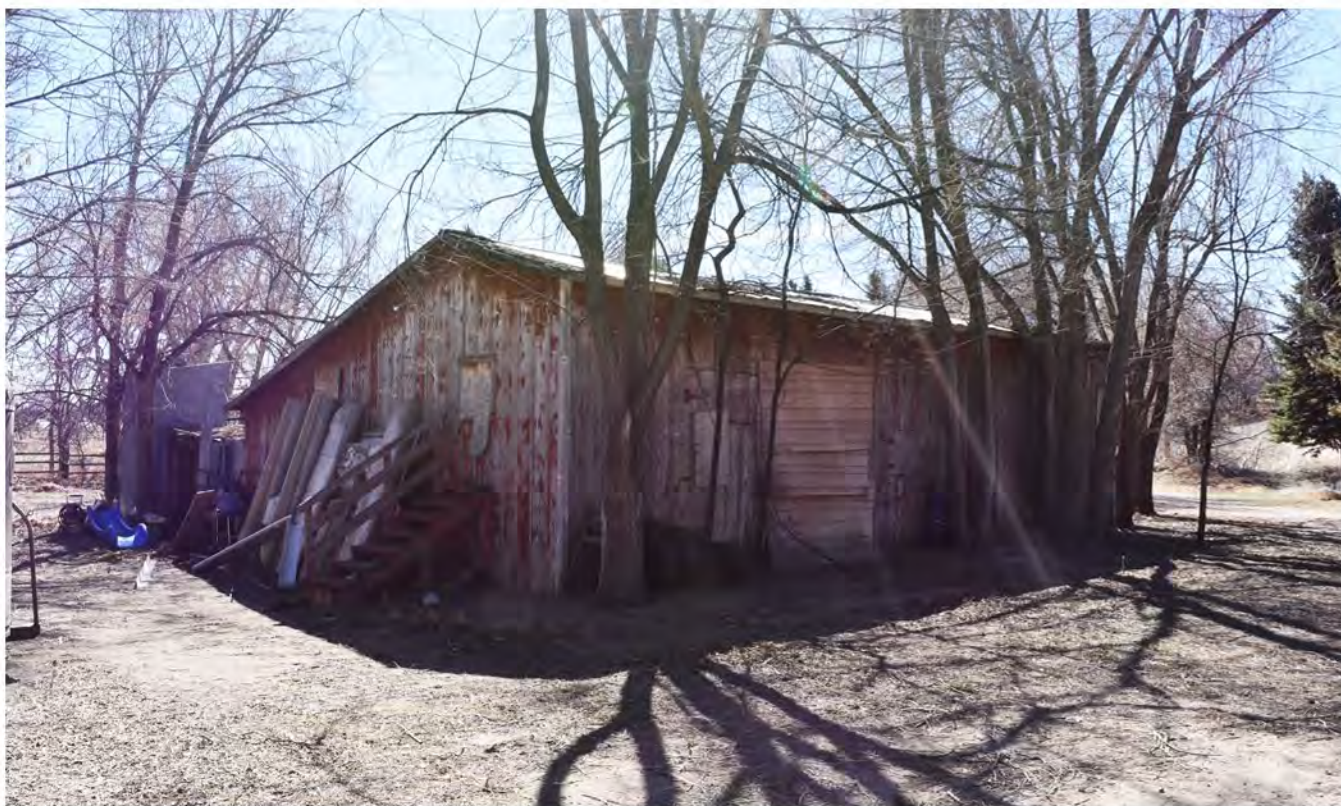
5LR14128_4: View south of one of two loathing sheds built in 1940. This one is located directly south of the 1930 concrete utility building seen in photo 3 above.
