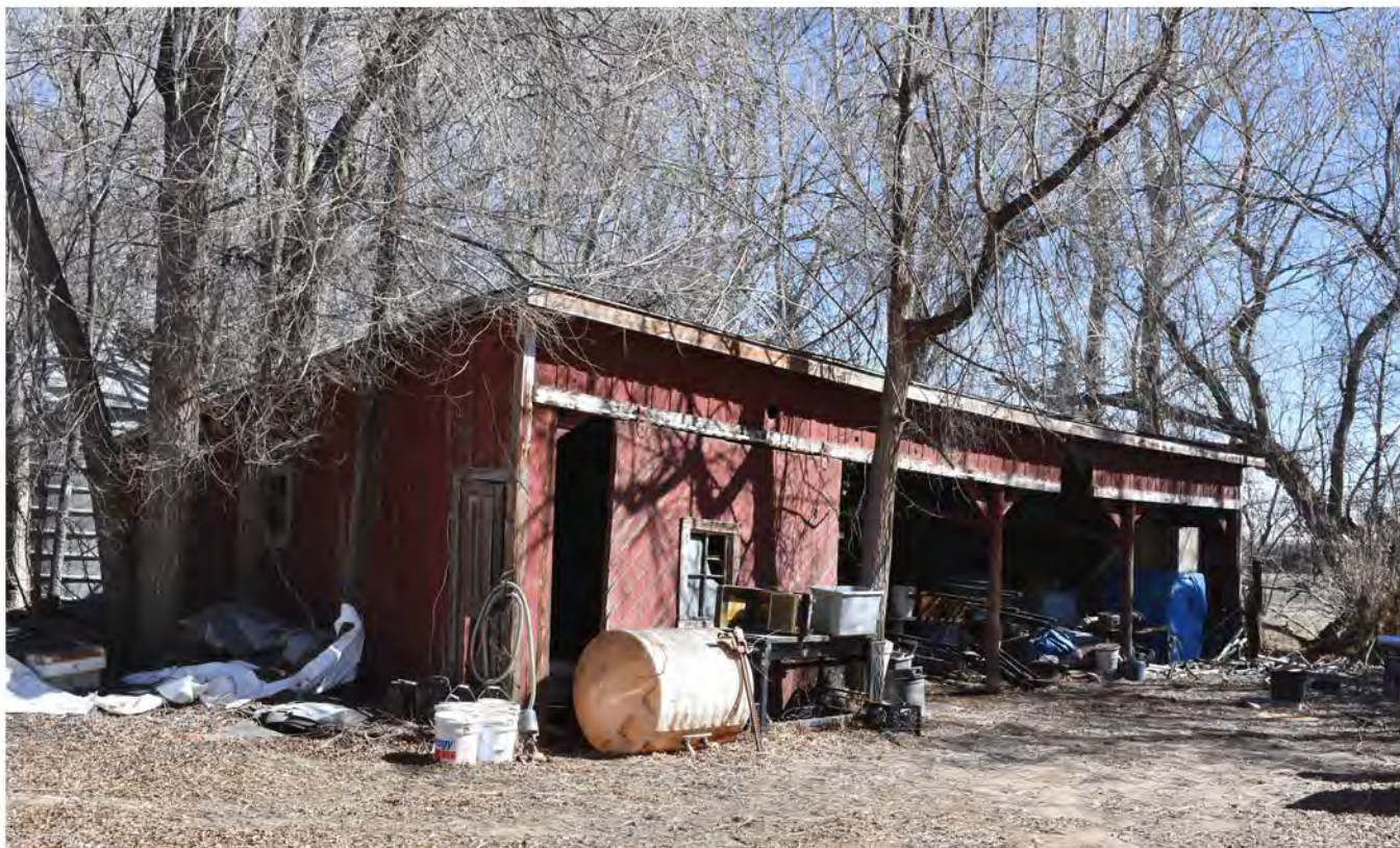
5LR14128_6: View east toward second loathing shed built in 1940, located just east of small shed/garage.
